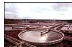
Water Purification Plant in Zelenograd (1998)
