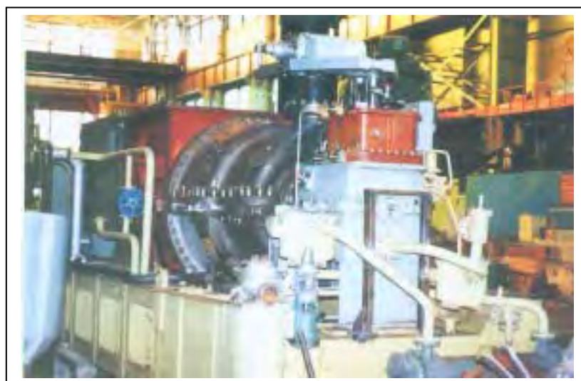
Tuman 4-K turbogenerator for the Verkhne-Mutnovskaya GPP
