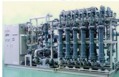
Semiconductor Polishing Wastewater (UF)
